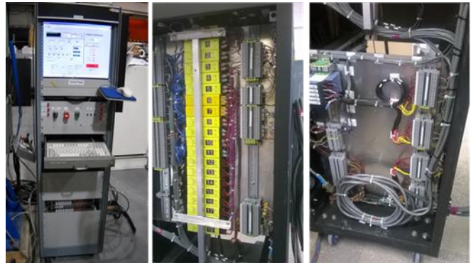
Fig. 7. Elements of advanced quench protection electronics developed at BNL for testing HTS magnets.
