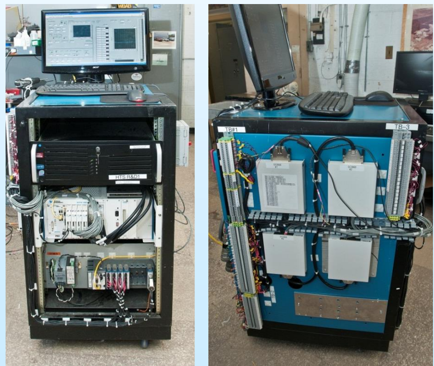
Cabinet #1 (32 channels, 1kV)
