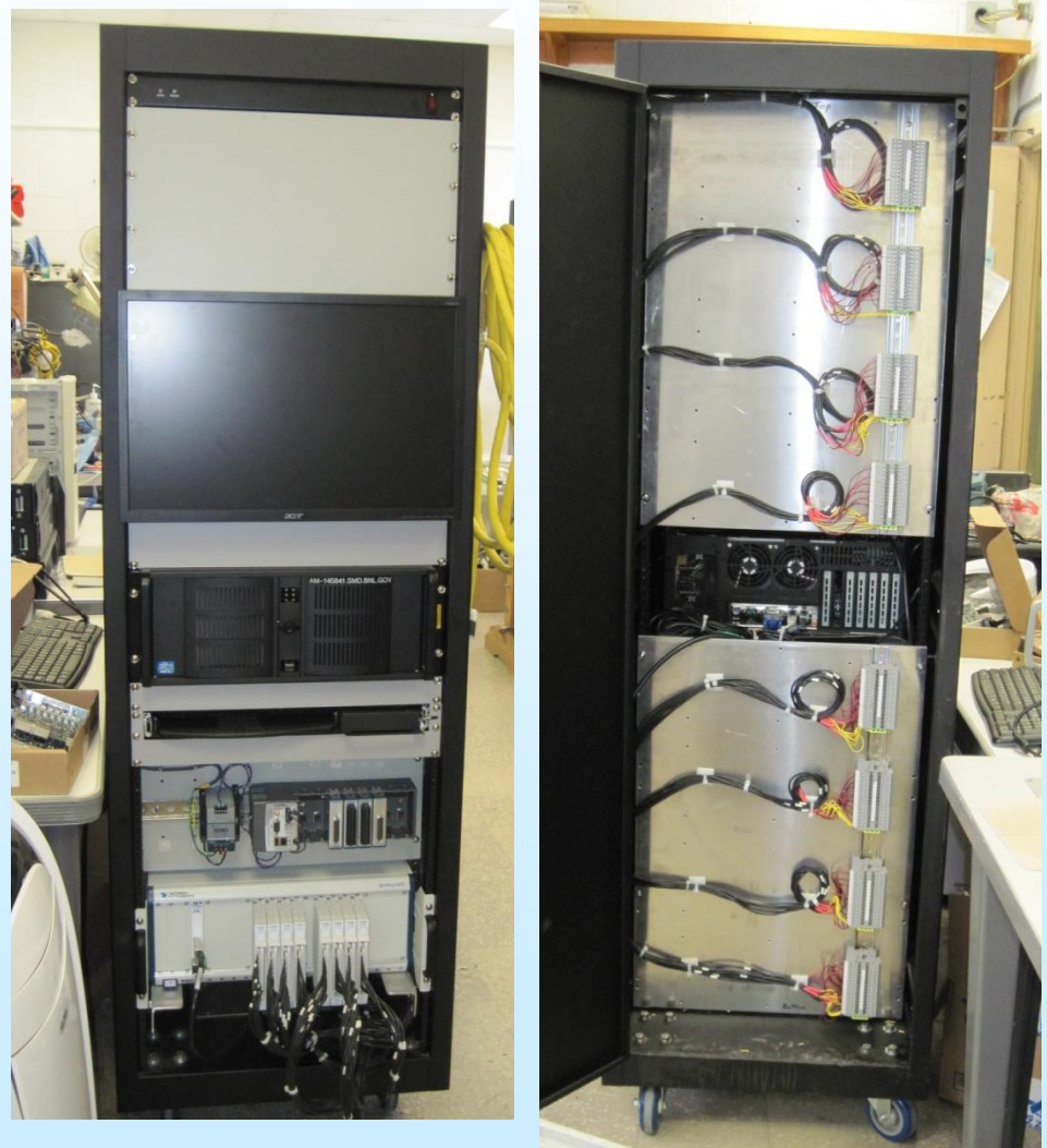
Cabinet #2 (32 channels, 1kV) (expandable to 64 and 3kV)
