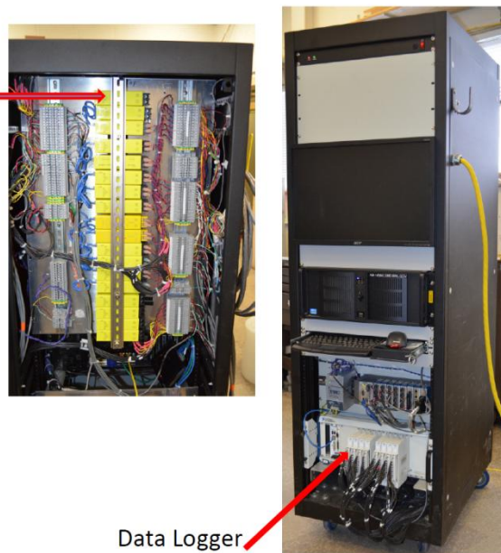
Fig.6: Quench Detection System (QDS) and Quench Protection System (QPS) hardware for inner and outer coil with a list of components including high voltage isolators.
