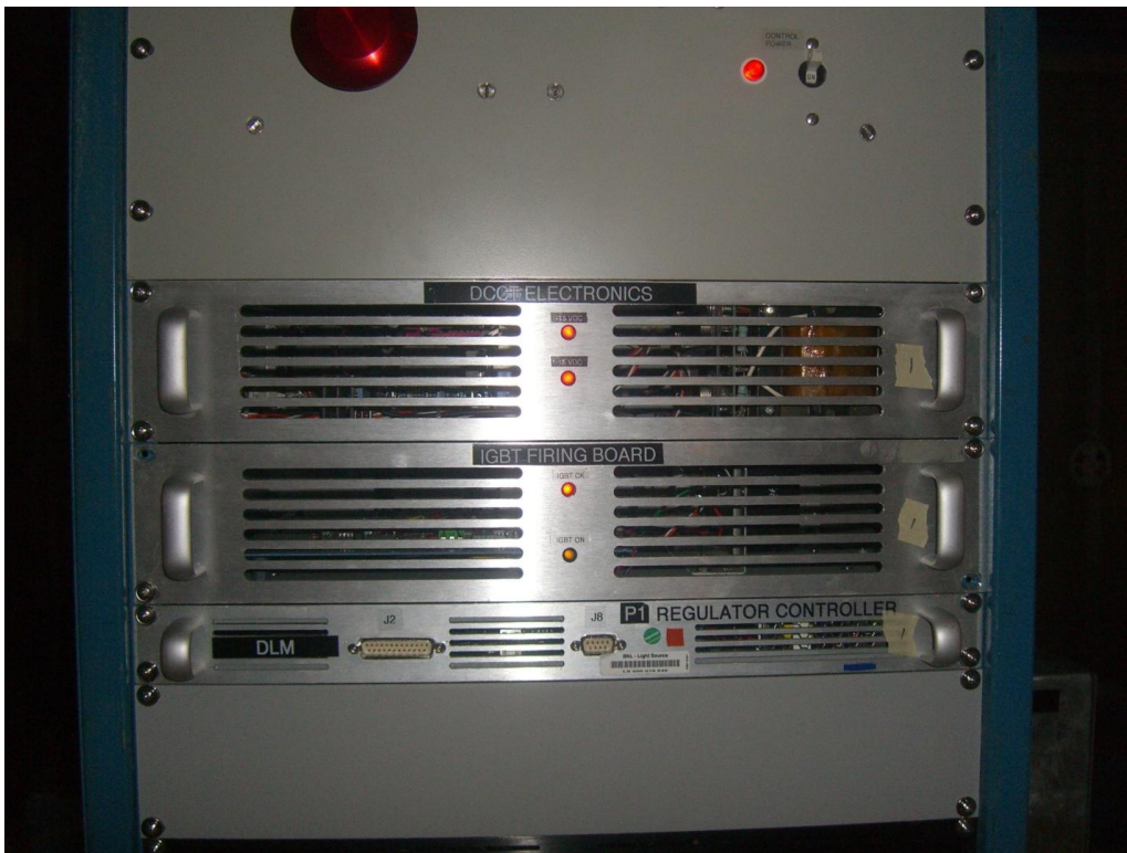
Figure 21: Power supplies for inner and outer coils.
